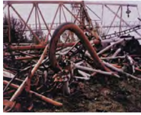
Fig. 17: 646 m mast in Poland after failure of a guy during exchange of guy ropes
